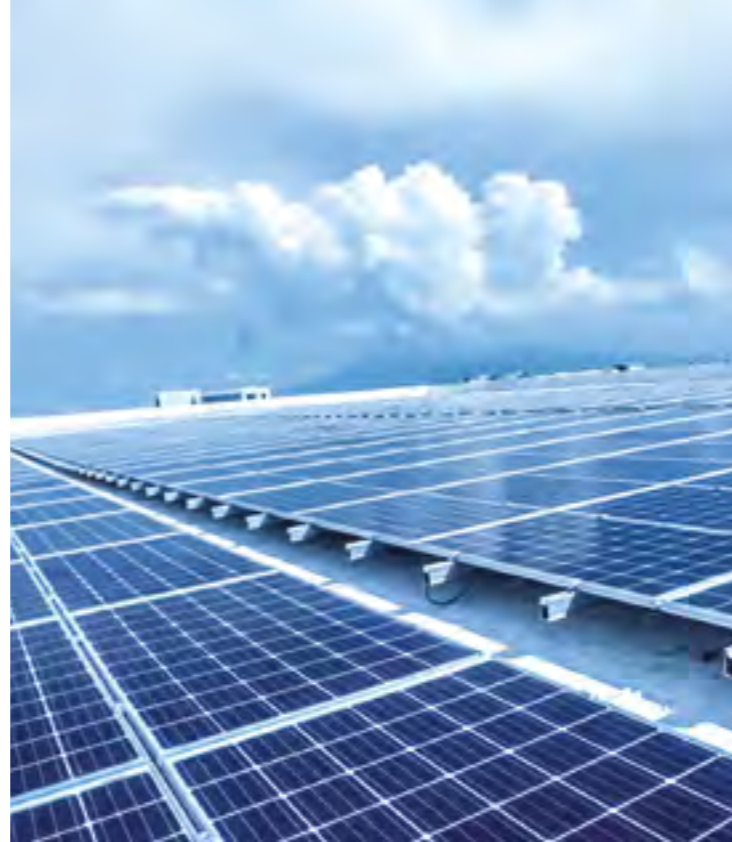
Solar electricity generation in our Batangas factory in the Philippines
