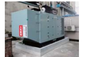
Self-power generator at the frozen-food manufacturer Sunburg
