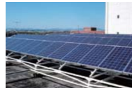
Solar panels at the Tokai Factory
